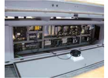
Electrical cabinet integrated into the basement
