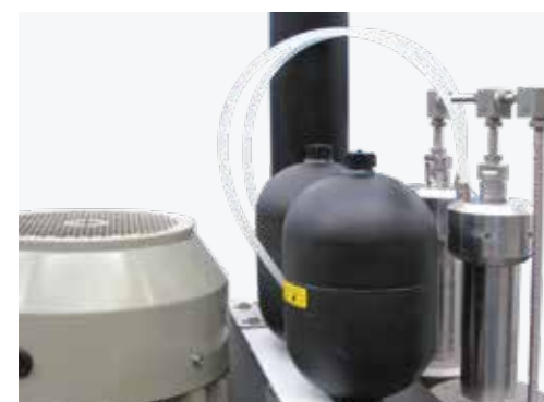
Nitrogen accumulator for managing the hydraulic cylinders return circuit
