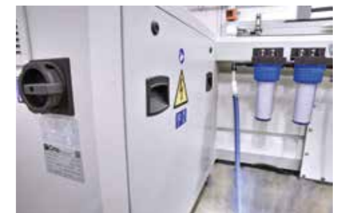
Control panel integrated into the base of the tank to reduce bulk on the ground
