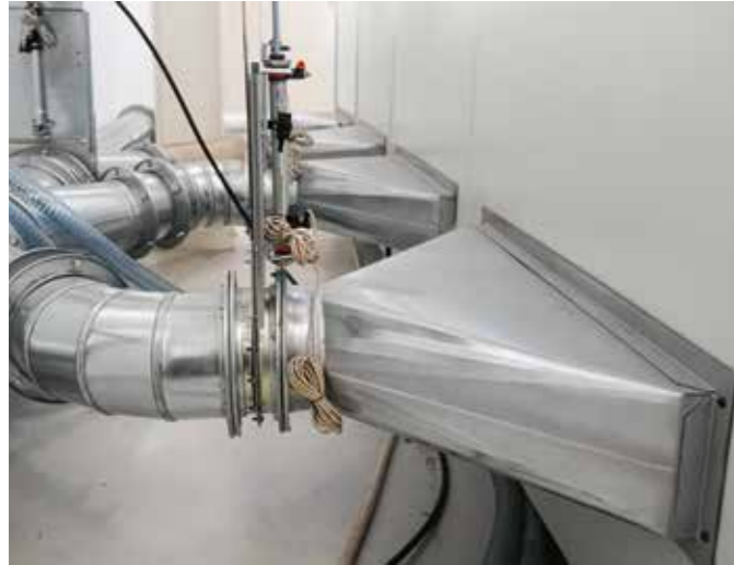
Dust extraction system for effective air change and dust abatement within the work area
